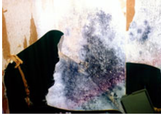
Photo 5: Mold growth behind wallpaper. Click on the image for larger version.
